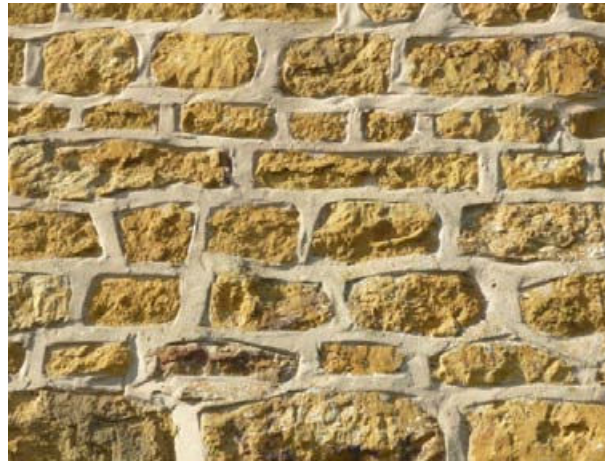
Ribbon or tuck pointing should be avoided as it causes the ironstone to deteriorate
