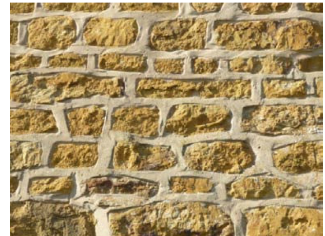
Proud pointing with cementaceous mortar can accelerate the erosion of the soft stone
