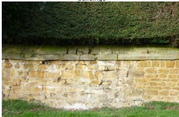
The effect of vegetation on boundary walls needs to be monitored
