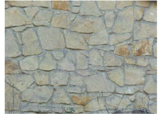
'Crazy paving' style stonework. Non local stone laid in non load bearing manner
