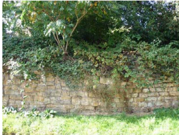
Condition of walls can be affected by vegetation
