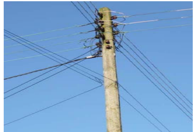
Visual impact of overhead wires
